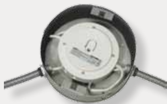
A hub shown inside the sealed junction box.
