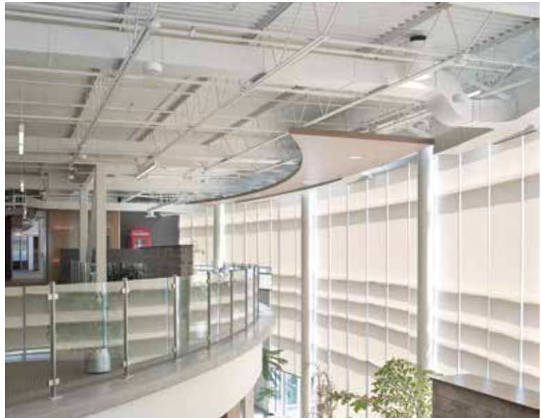
Hubs and loudspeakers suspended in an open ceiling.
